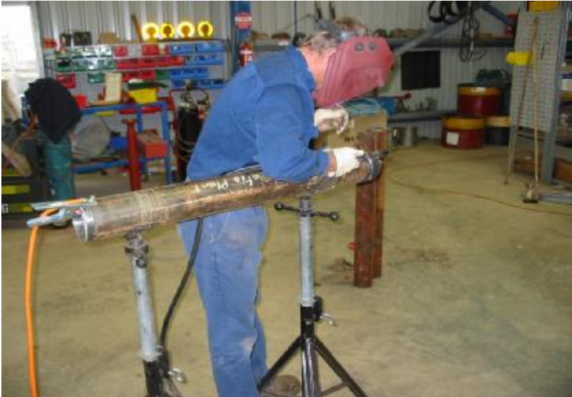
A simple photo showing the skills adopted from some coaching and mentoring in the cleaning, set up, technique, weld sequence, transferring of identification marking and sequence of weld passes on a small pressure component for the oil and gas industry.
